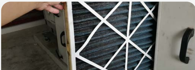
COMPRESSED AIR FILTER
